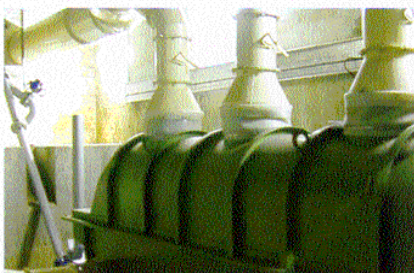
Metallurgical Coke Fluid Bed Cooler
